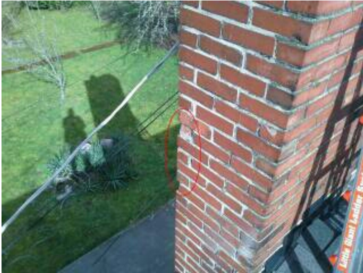
some brick spalling
