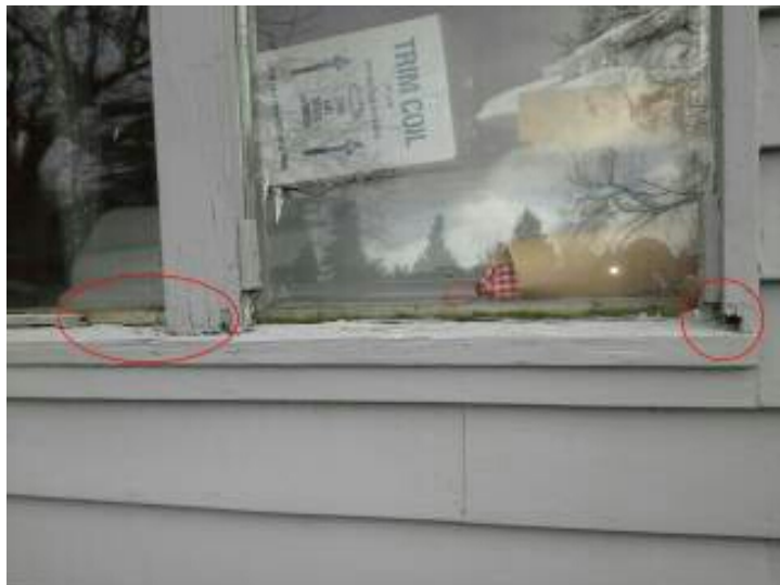
wood rot present at rear of garage
